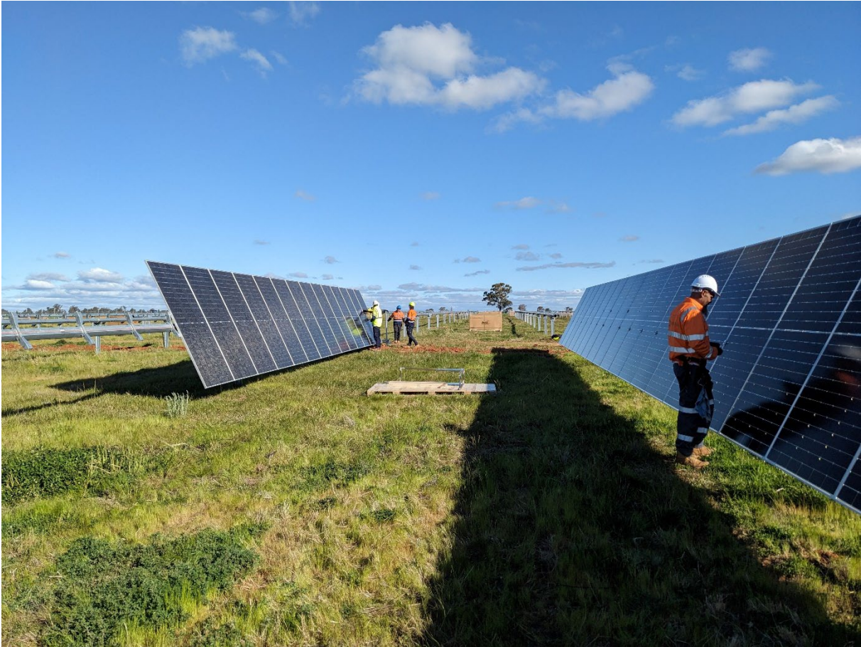
Photo Courtesy of Komo Energy – construction progress at the Grong Grong Solar Farm.
